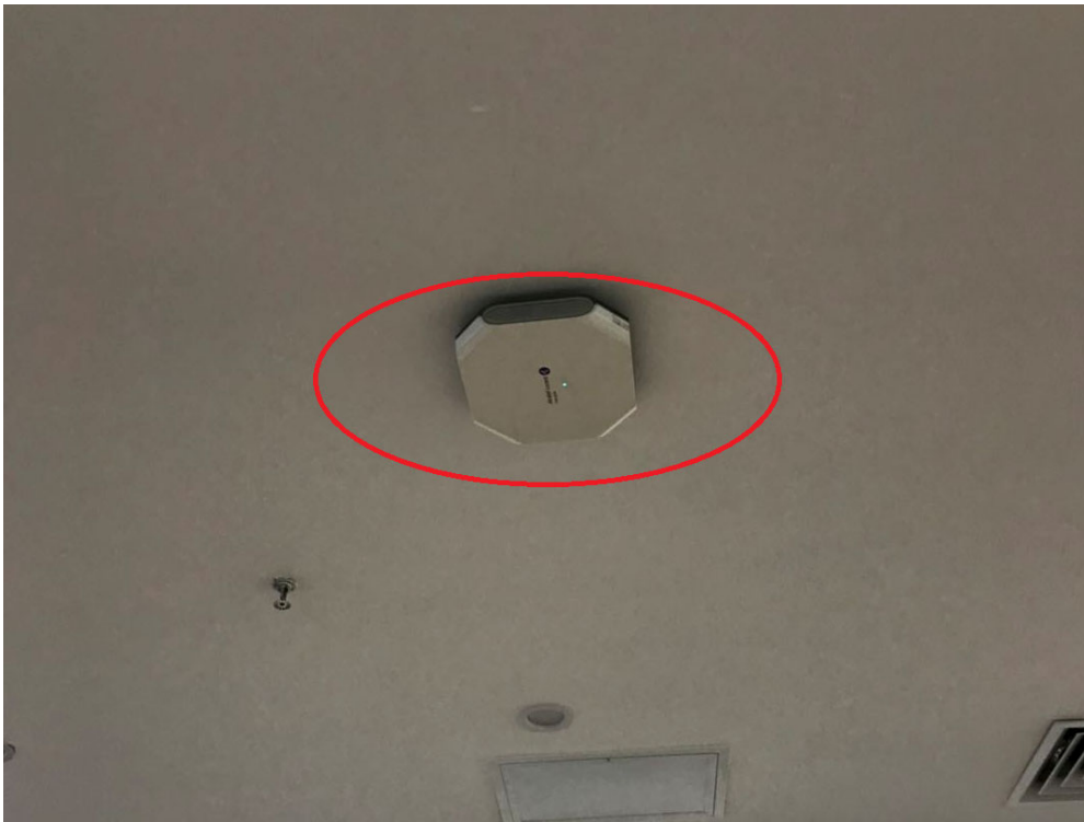
Figure 12: AP ceiling mount in conference hall
